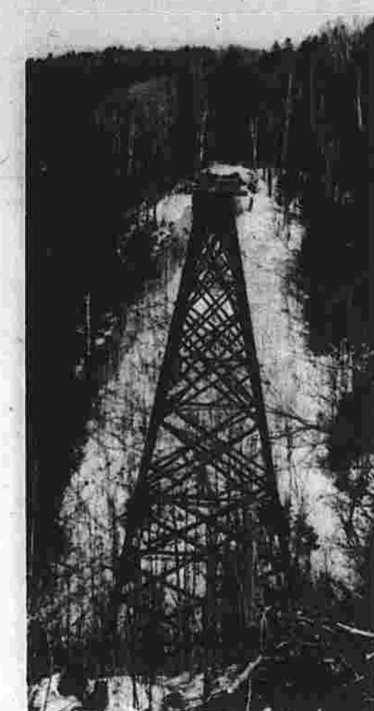
Landmark being dismantled A landmark of a bygone era will be coming down shortly as workers prepare to dismantle the Somerset Railroad trestle near Bingham, Maine, which was built in 1904. The 125-foot tall trestle spanned 700 feet across the Gulf Stream to carry summer people from Boston and New York to vacations in Moosehead Lake and the Hotel Kineo. It was last used by pulp trucks hauling logs to pulp mills in 1936. (UPI photo)
